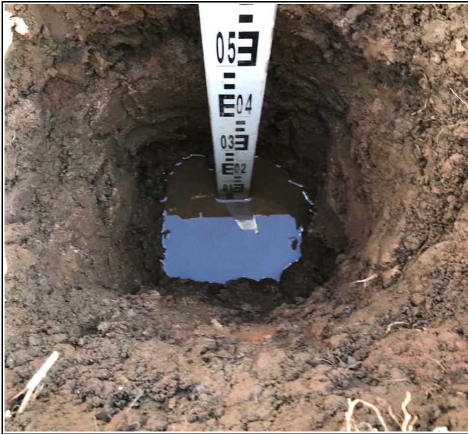
Plot 95 Showing Membrane Placement (Below Water Ingress)
