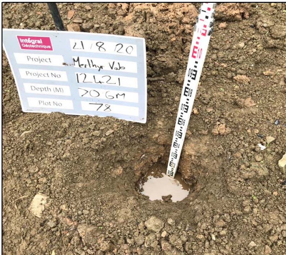
Plot 78 Excavation Trial pit Membrane Present (Water Ingress)
