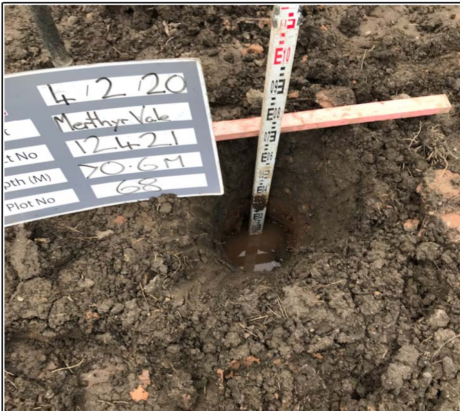
Plot 68 Excavation Pit with Membrane at Base of Soils (water Ingress)
