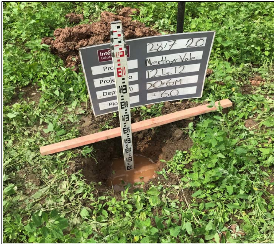
Plot 60 Excavation Trial pit Membrane Present (Water Ingress)
