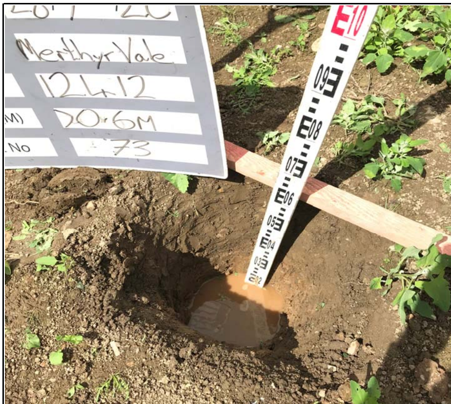
Plot 73 Excavation Trial Pit Membrane Present (Water Ingress)
