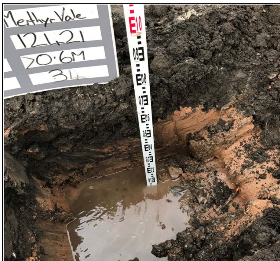
Plot 34 Membrane Exposure ( High Water Ingress)
