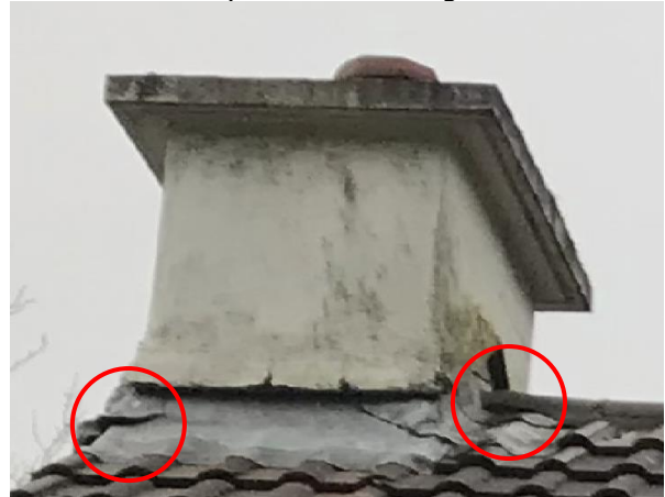
Photo 2: Chimney and Raised Ridge Tile
