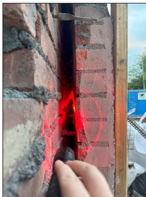
Plate 4 – The cobwebs within the cavity walls.
