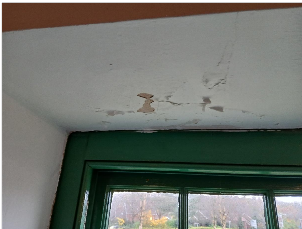
Plate 39. Example of peeling paint near window in main room on ground floor of No. 4 Chapel Row, looking west-southwest.
